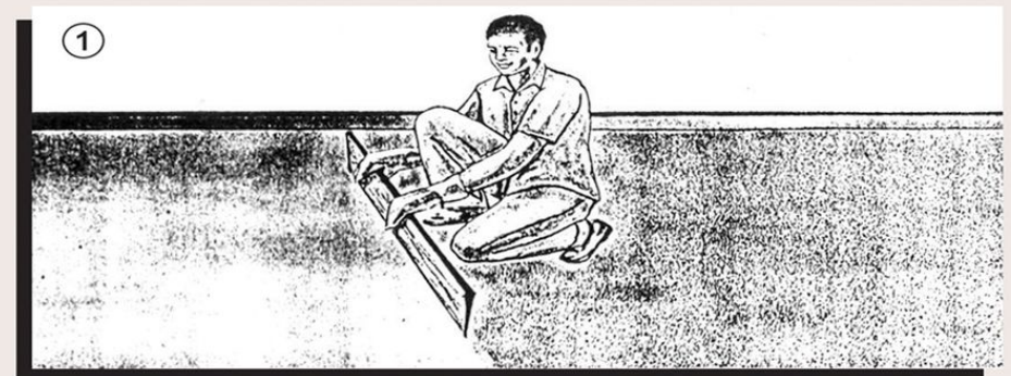
For Pavers: Spread Sand on the area to be laid on an average of 50mm thickness, Compact and screed the sand
